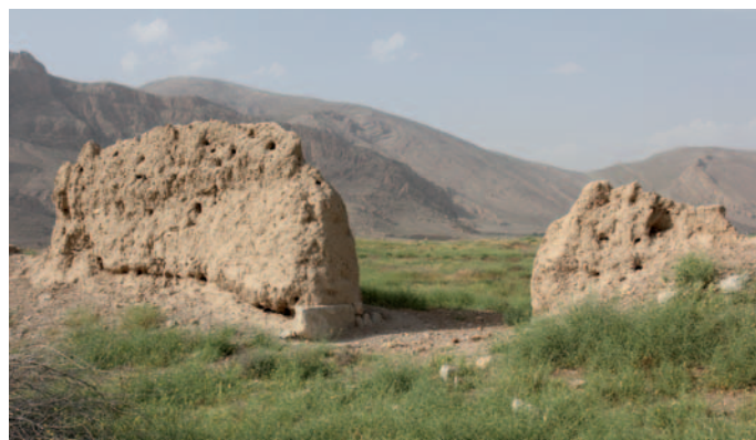
Fig. 1. A 19th century square enclosure, with mud walls on a small stone foundation, known as takht-e tavus (the peacock throne; photo M. Rugiadi)
